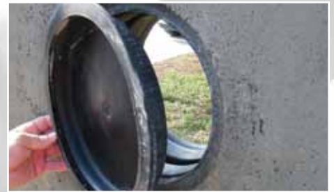
6. After concrete is cured, pry off the locator caps with a pry bar.
